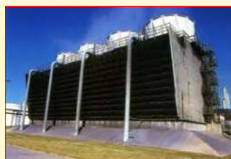
Cooling Water Chemicals
